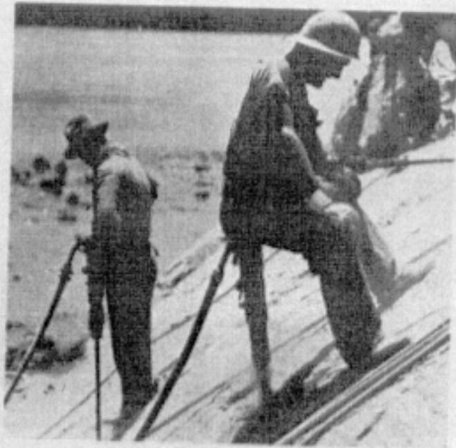
This worker varied standard approach to jackscrew techniques to get the job done.
